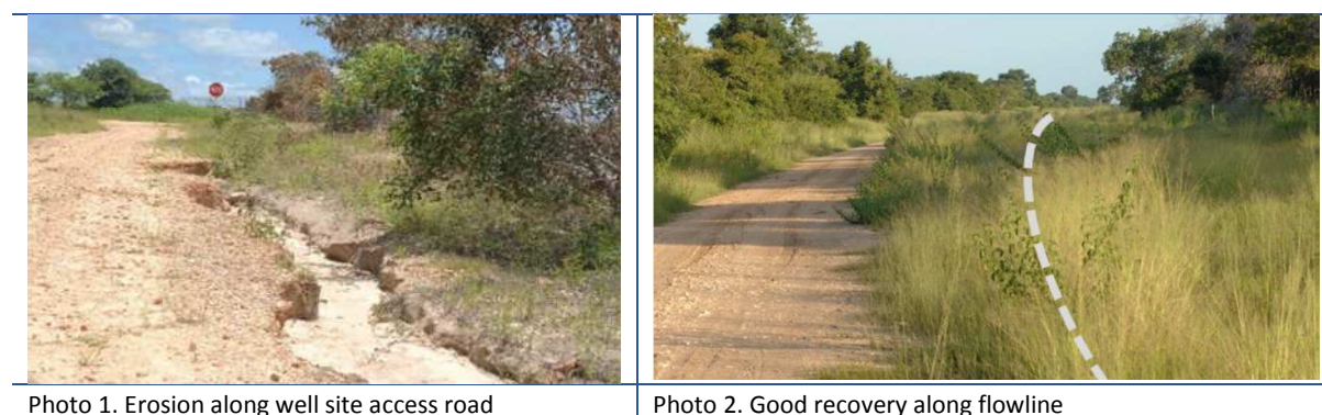
Photo 1. Erosion along well site access road
